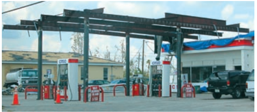
A gas station lost its roof during Hurricane Charley.
